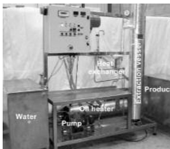
Figure 5: Photograph of the pilot plant
