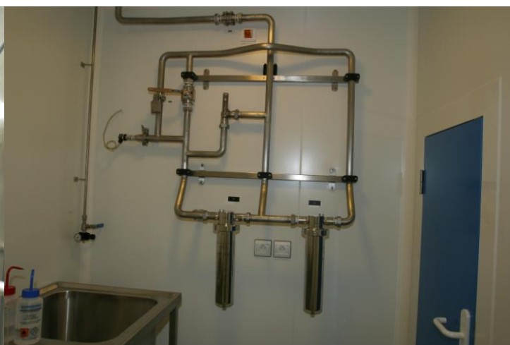
Figure 2: Effluent filtering system
