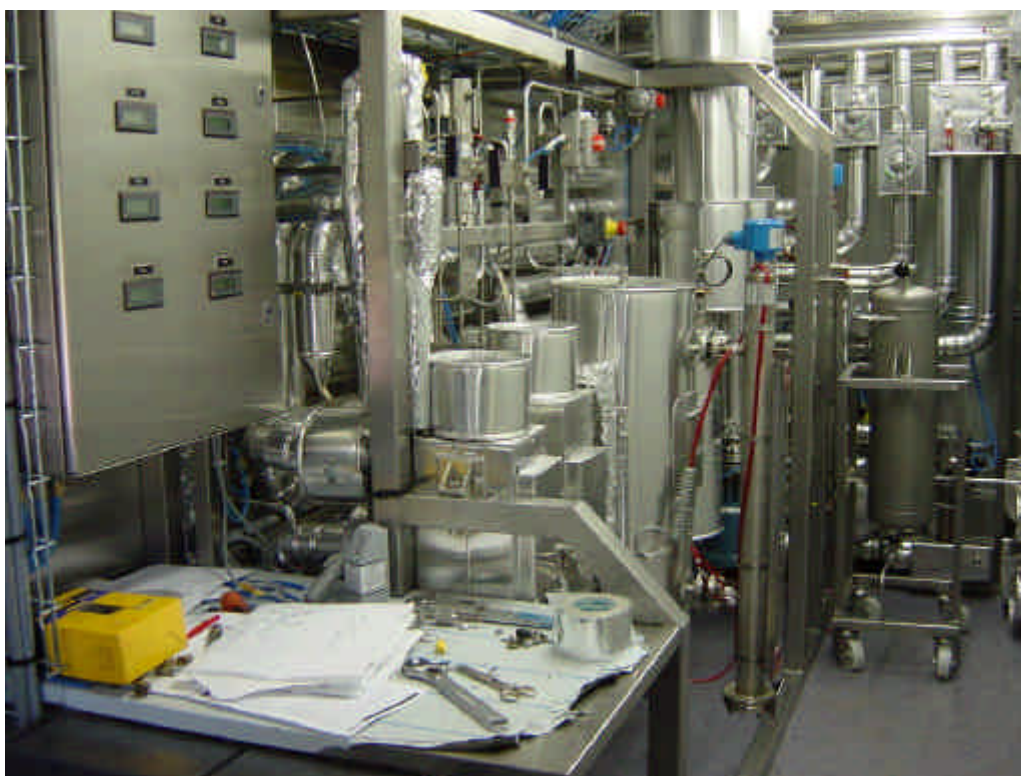
Figure 3. The reactors, the flash drum and the bottom of the distillation column in the pilot plant at Härröd Research.
