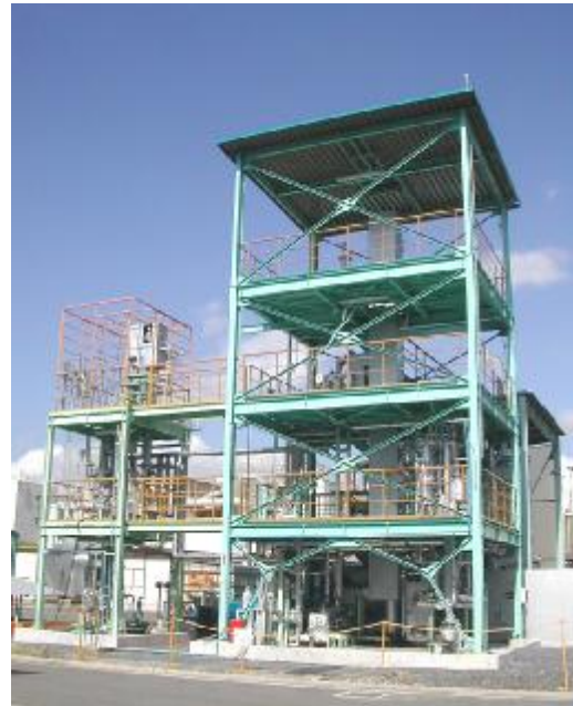
Fig.8 The Bench Test Plant
