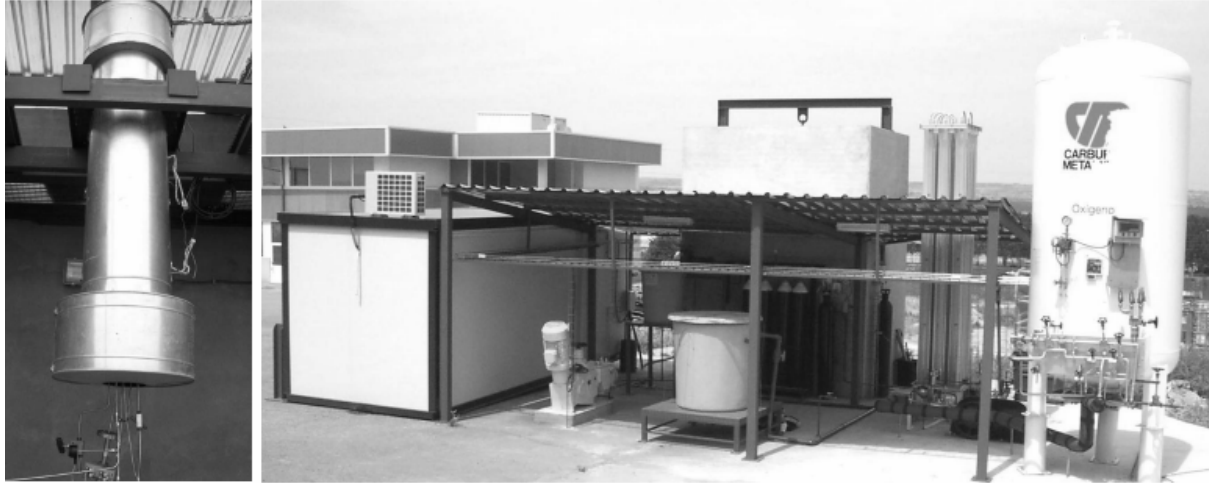
Figure 7: Picture of the SCWO demonstration plant
